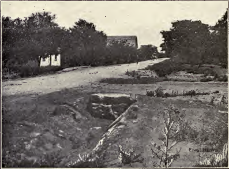
FIG. 5.—DEEP DITCH AND CULVERT PARTIALLY FILLED WITH DIRT WASHINGS
